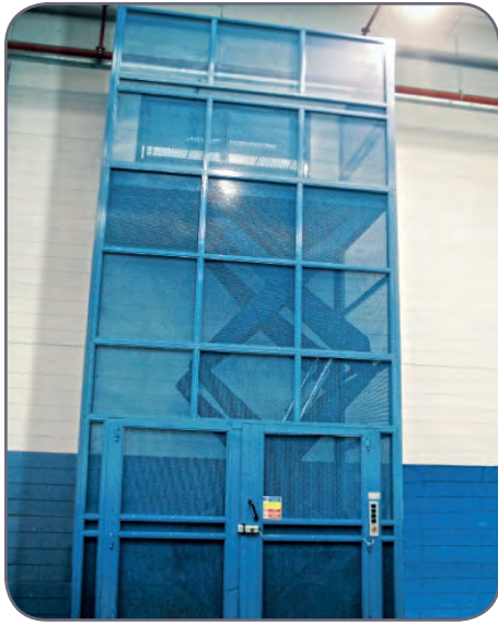
lift connecting two floors
